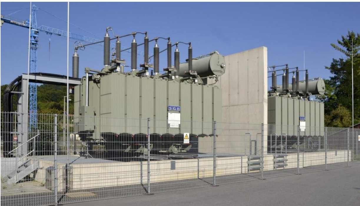
Plate 4.2 Transformer – typical appearance with a concrete fire wall and a plinth
