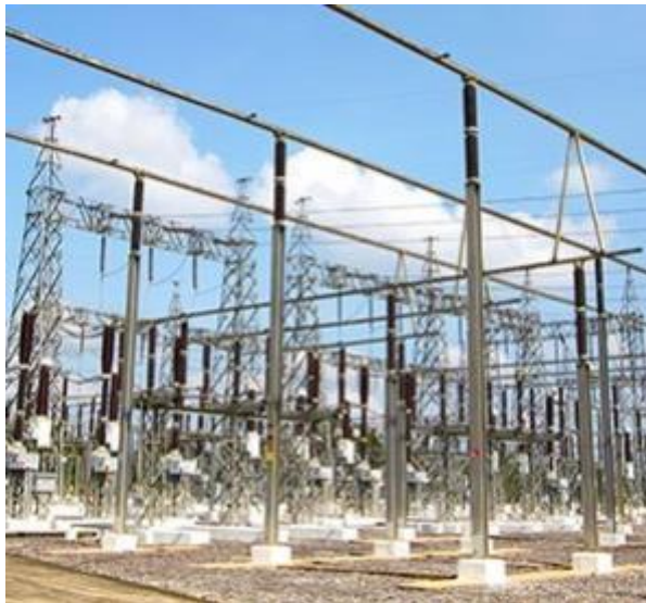
Plate 3.1 Typical AIS external switchgear (400kV single busbar)
