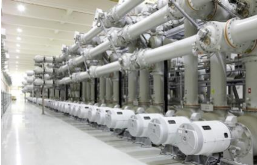
Plate 3.2 Typical 400kV GIS switchgear
