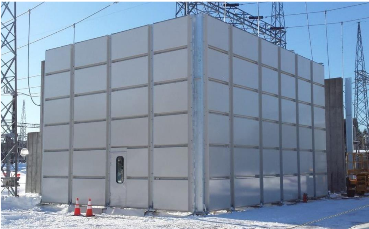
Plate 4.4 A typical steel panel noise enclosure surrounding a transformer.
