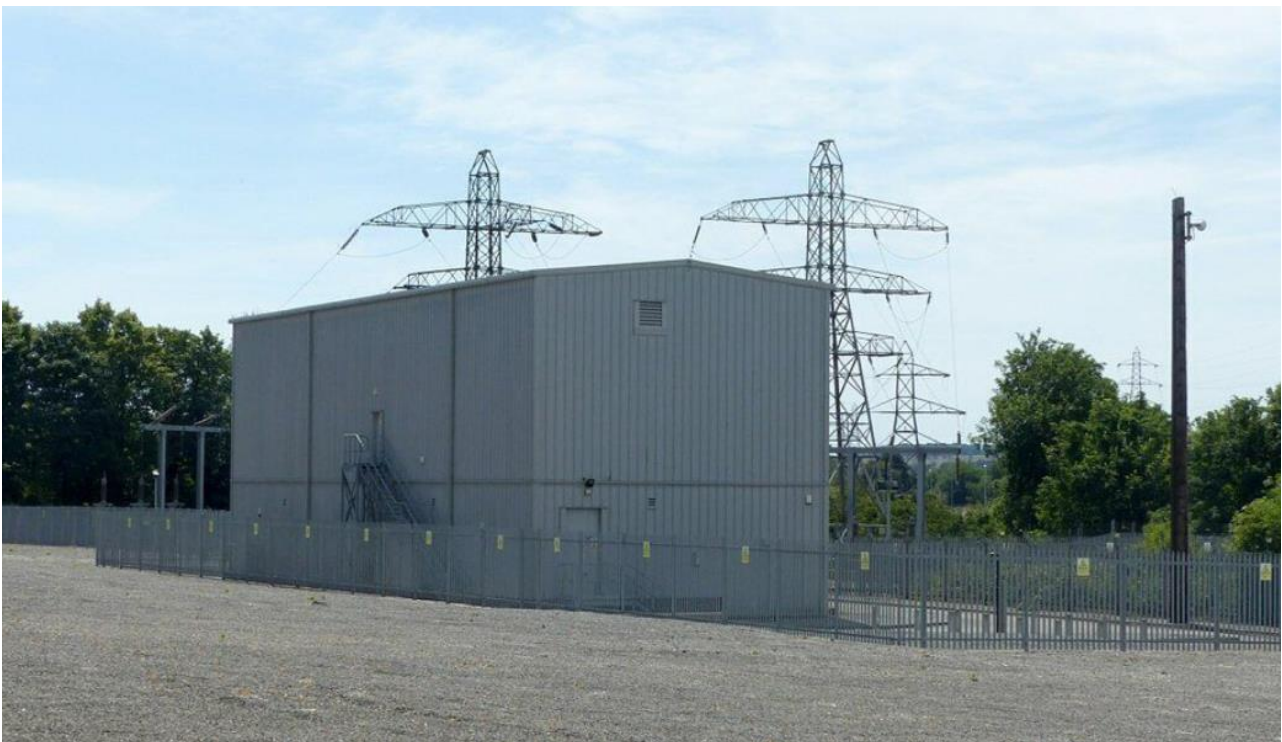
Plate 4.1 Typical GIS building without a control room annexe
