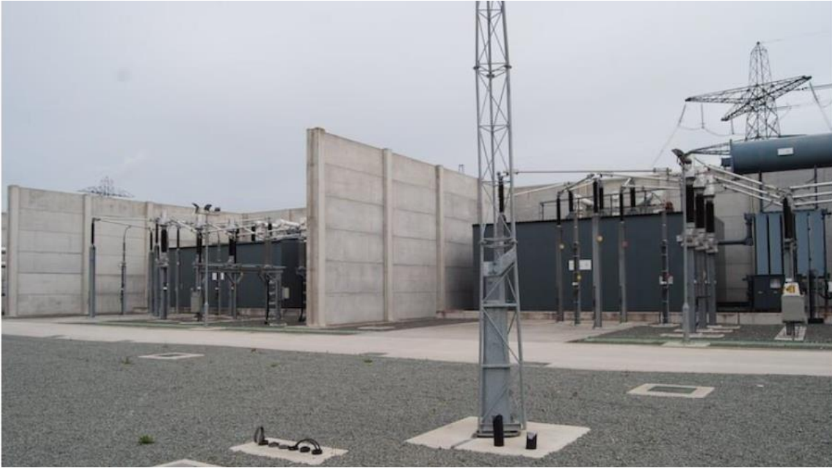
Plate 4.3 A typical transformers in acoustic enclosures (grey metal boxes) with concrete fire walls
